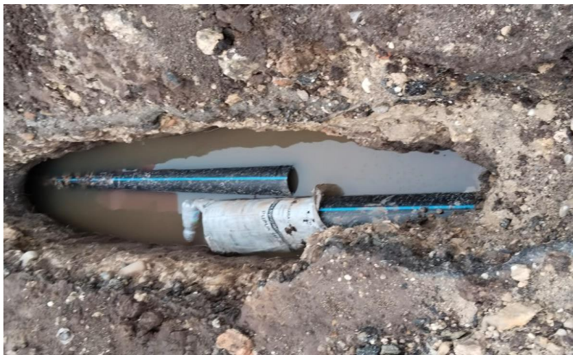
Figure 6. Underground pipe installation connection on Jl. Arjuna RW 08 and 09, East Labuh Baru, Pekanbaru
