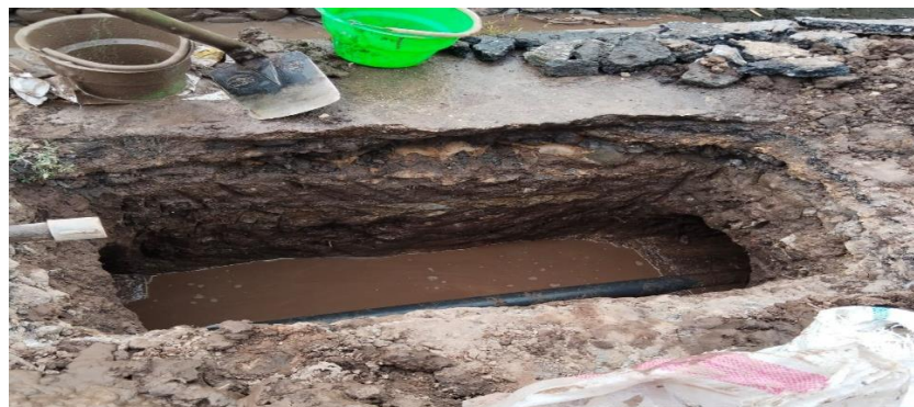
Figure 4. Pipe installation connection with overflow due to flooding
