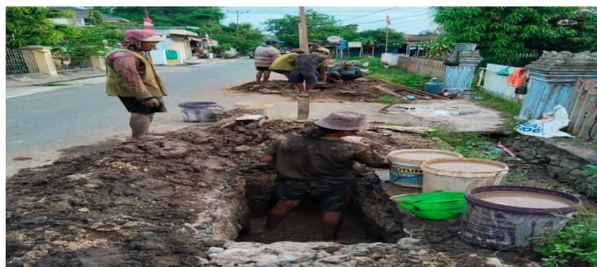
Figure 2. Excavation work with dimensions of 1 meter \times 80 cm on Jl. Arjuna, RW 08 and 09, East Labuh Baru, Pekanbaru
