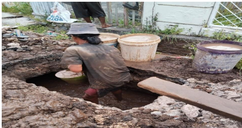
Figure 3. Drainage of water from the excavation site to a different location on Jl. Arjuna RW 08 and 09, East Labuh Baru, Pekanbaru
