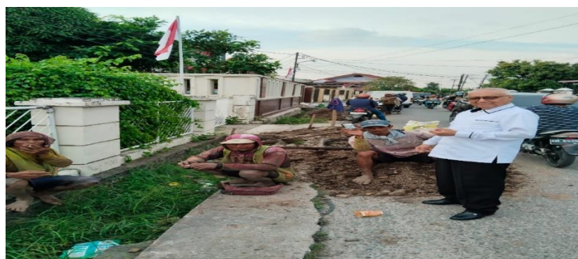
Figure 7. Community service team coordinating with workers on the installation of PDAM pipes on Jl. Arjuna RW 08 and 09
