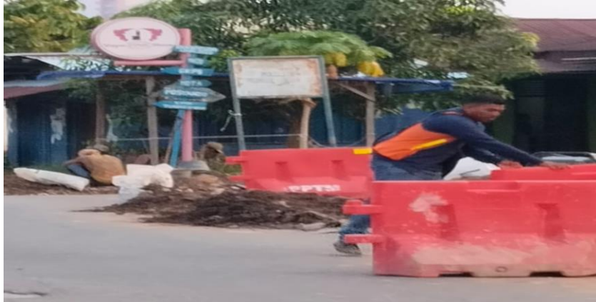
Figure 5. Traffic management during pipe installation on Jl. Arjuna RW 08 and 09, East Labuh Baru, Pekanbaru
